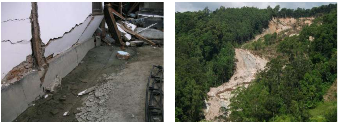
Figure 3.13. The left figure: Liquefaction caused damaged to residents' houses due to the earthquake on September 28 th , 2018 in Panau Village, Sigi Biromaru District, Sigi Regency. The right figure: Landslides and flow-type andslides threaten residents of Sungku Village, Kulawi District, Sigi Regency.
